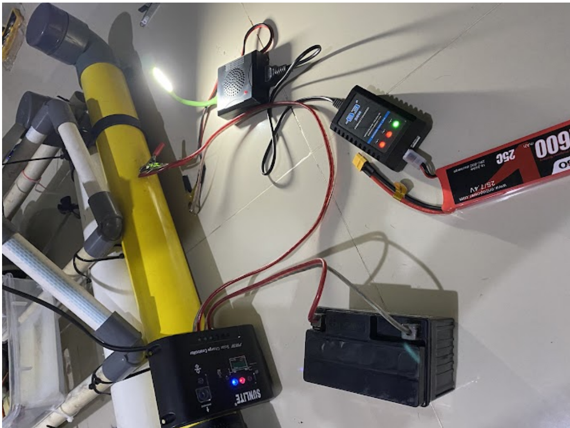
Picture 4.1.1 Testing electrical system after battery is fully charged
